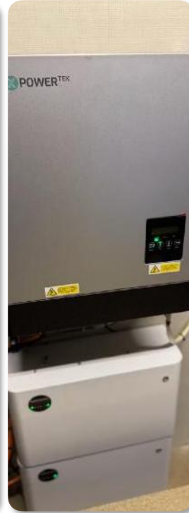
Building management systems
