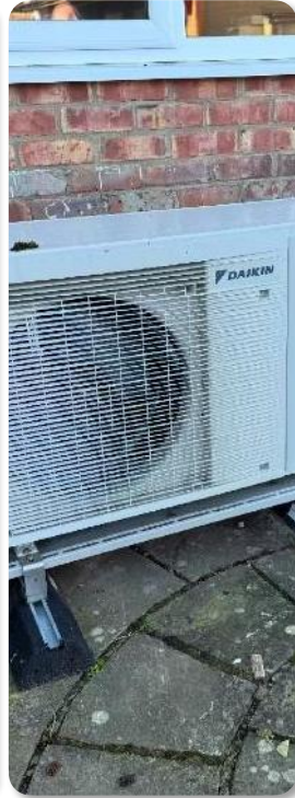
Air source heat pump
