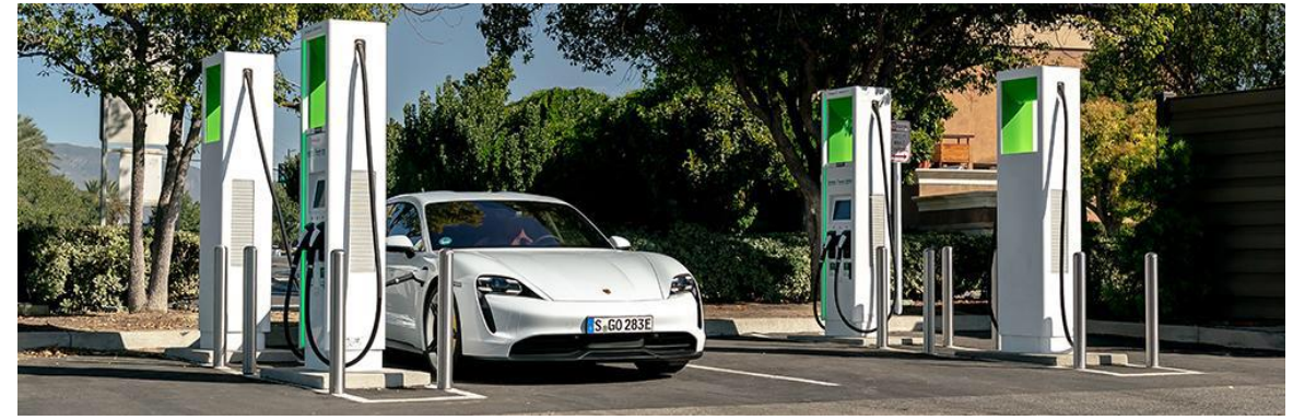
Destination, On Route & Charging Hubs
