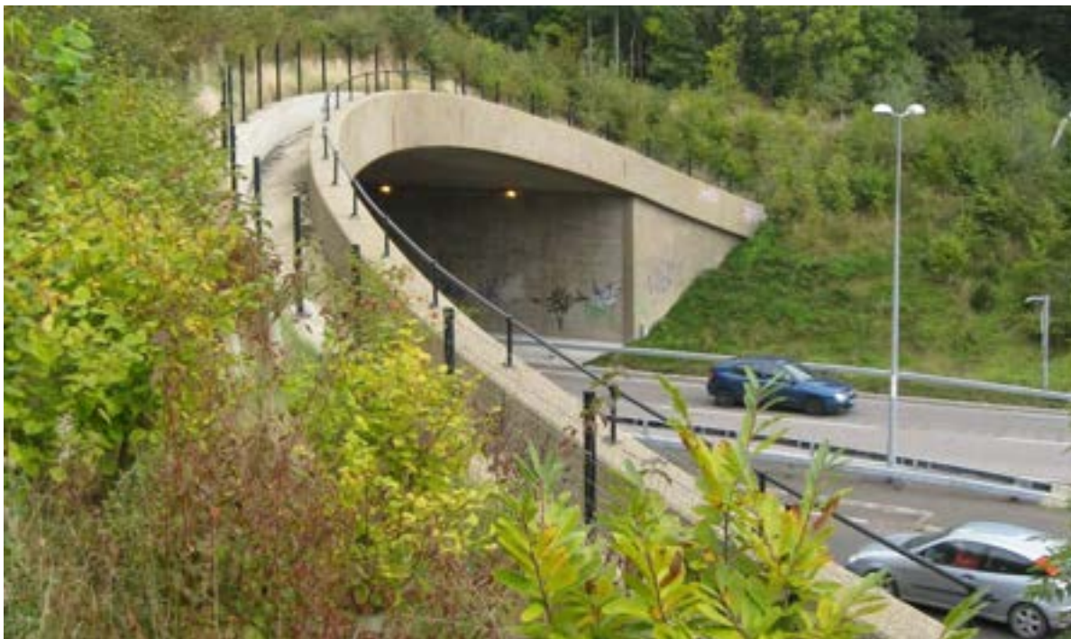
Scotney Castle Land Bridge on the A21 in Kent [Image courtesy of Fira 6 ]
