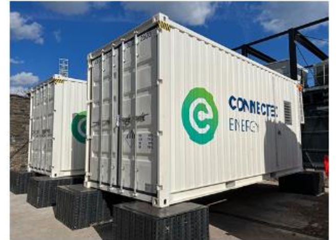
Battery storage containers
